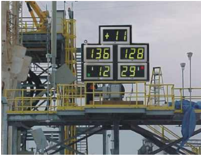
Figure 2. Large digit display within hazardous area.
