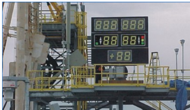
Figure 2. Large digit display located within a hazardous area in an oil terminal.
